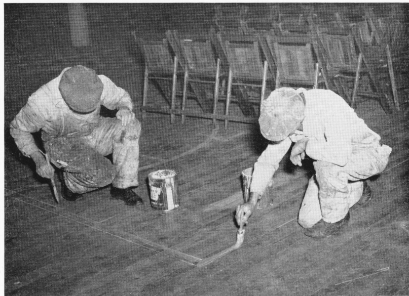
William Turner and James Pedin are shown here marking off the floor for badminton and other games requiring large floor space. This is the main room of the hall, and is to be the recreation hall in the near future. Pipes will be covered in this room and permanent benches installed around the hall for spectators and contestants. Scovill has approved. It's up to Washington now.
