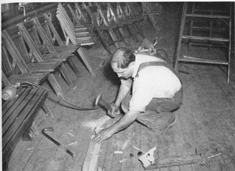
New floor boards were needed in Doolittle Alley Hall, and in they go. Carmine Cocchiola, carpenter, beats nails into submission, later to countersink them. Pictures on this page are only cornerstone repairs compared to the extensive plan Scovill has approved for remodeling. Recreation will get off to a new start in spacious new quarters.
