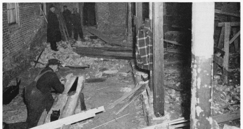
To prepare for the rolling cafeterias soon to feed Scovill employees, the old Spoon Shop on Silver street gets a rebuilding job. In the upper photo, Frank Argenta and Saverio Guerrara, bricklayers, put in a doorway with Salvatore Dadonna, their helper. Lower photo: In the rear, Supervisor Tom Fleming watches the procedure, and in the foreground Lee Garrigus makes repairs on a door casing. This is where the kitchen will be situated.
