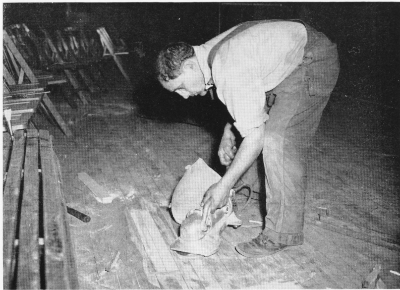
Carmine again, here with a sander. The men are making sure that this section of the floor is positively smooth, with no chances of splinters or ridges to interfere with activities. The Company is awaiting a priority order from Washington before complete plans can be realized. Men here make repairs that can now be done with materials available.
